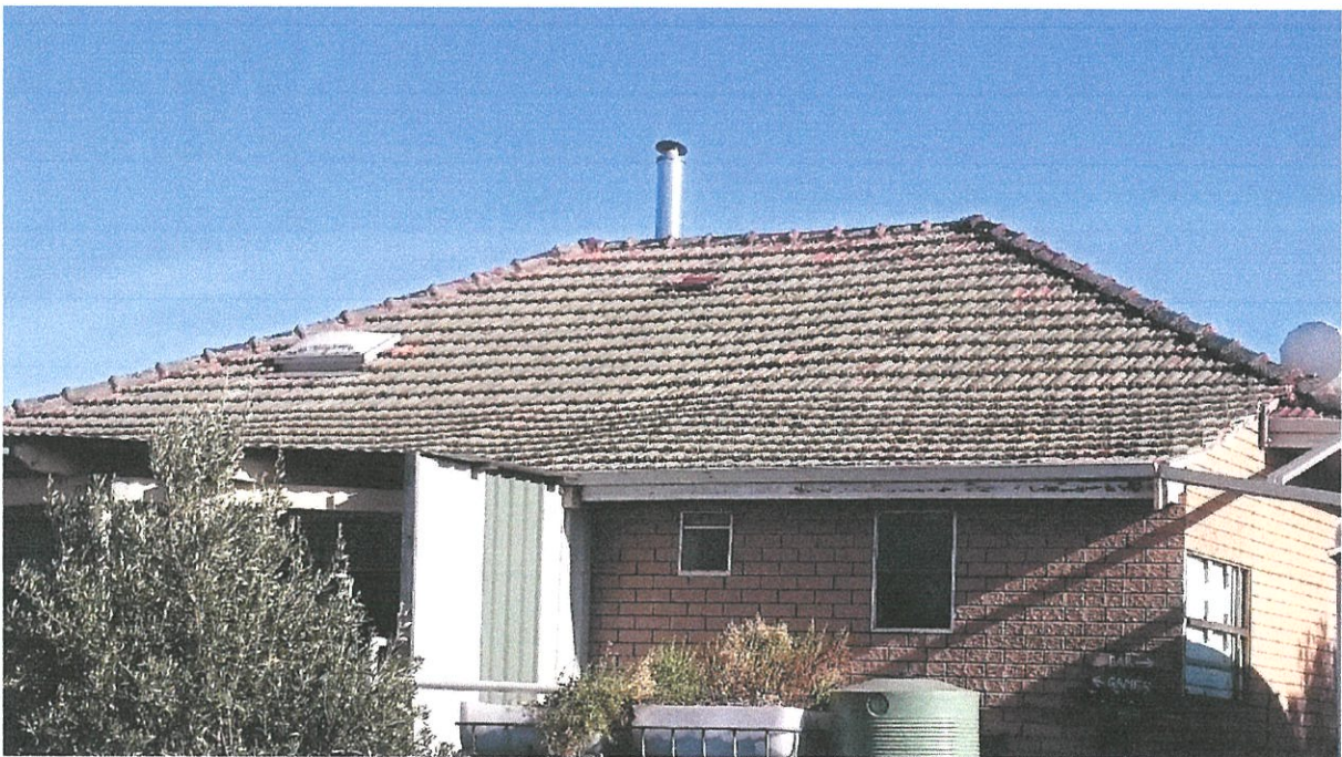
Sagging roof on the Eastern side.
