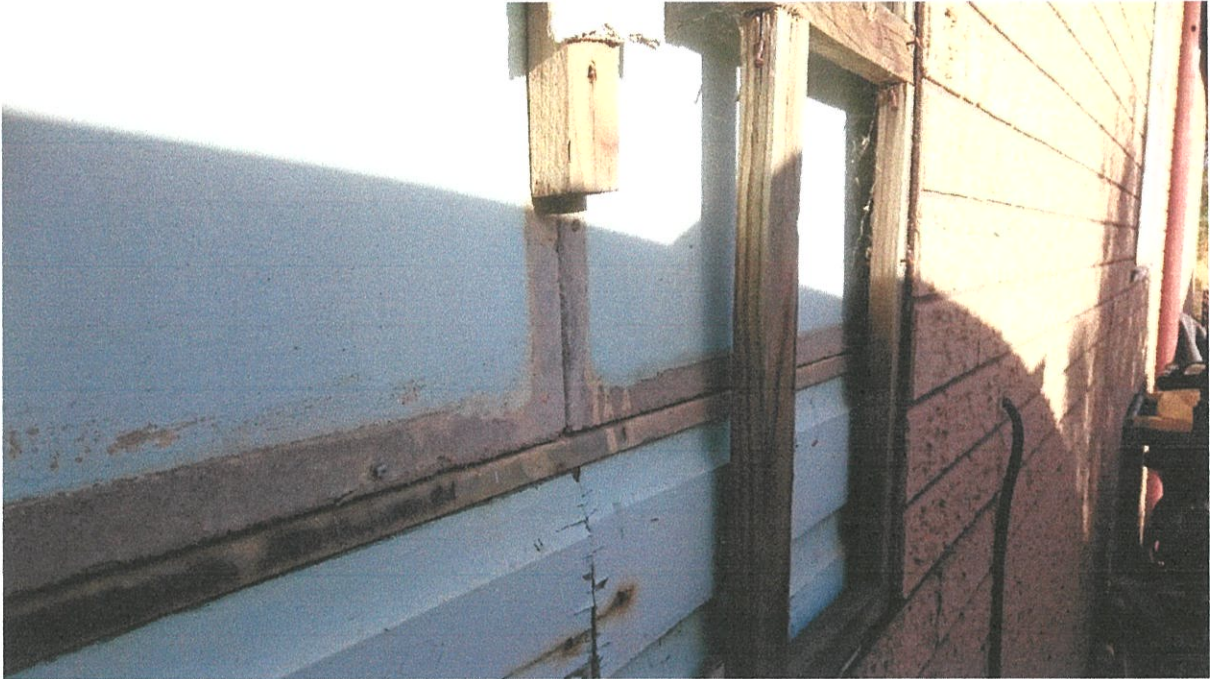
The bottom of the original wall is weatherboard the top is asbestos sheeting with raw unpainted edges.
