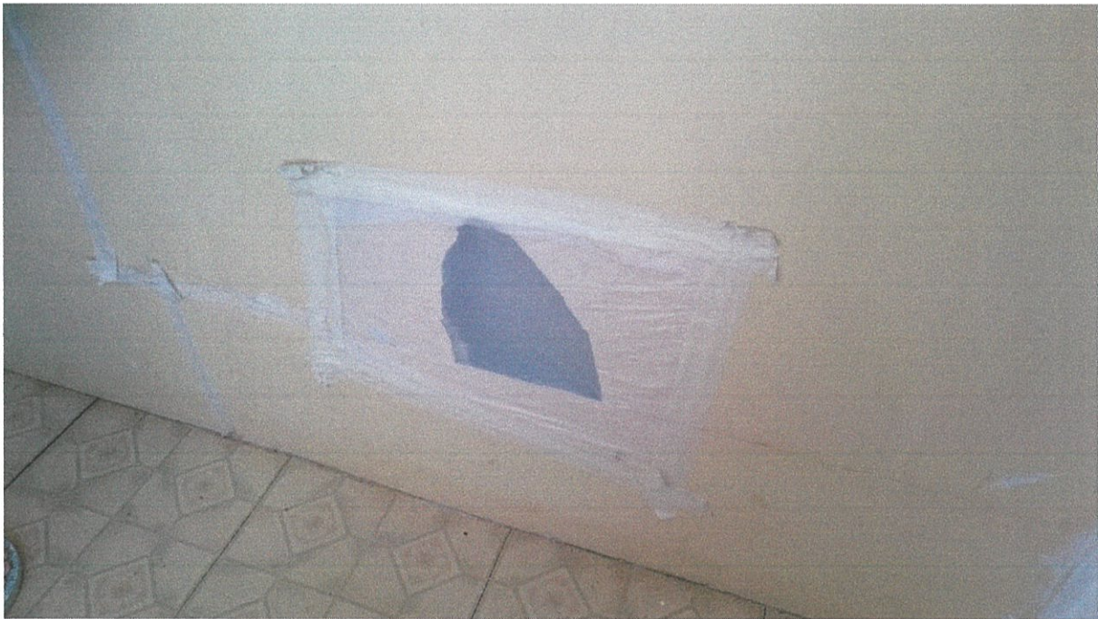
Hole in asbestos sheet in the bathroom.
