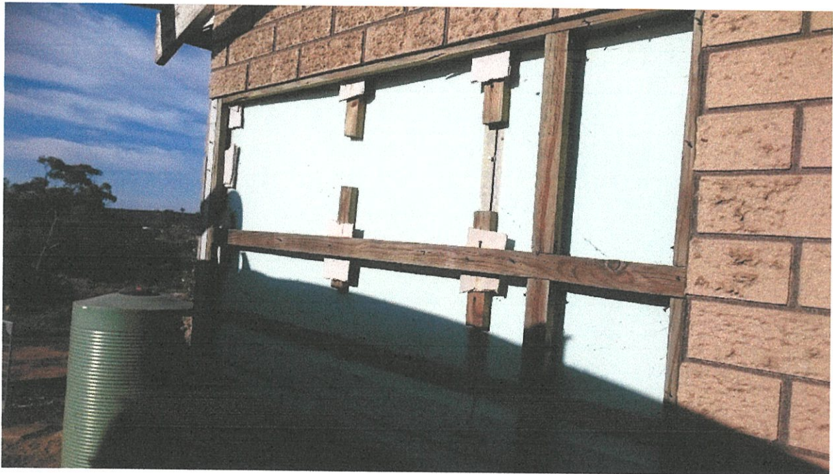
A fake brick panel has come away revealing timber and broken asbestos packers beneath.
