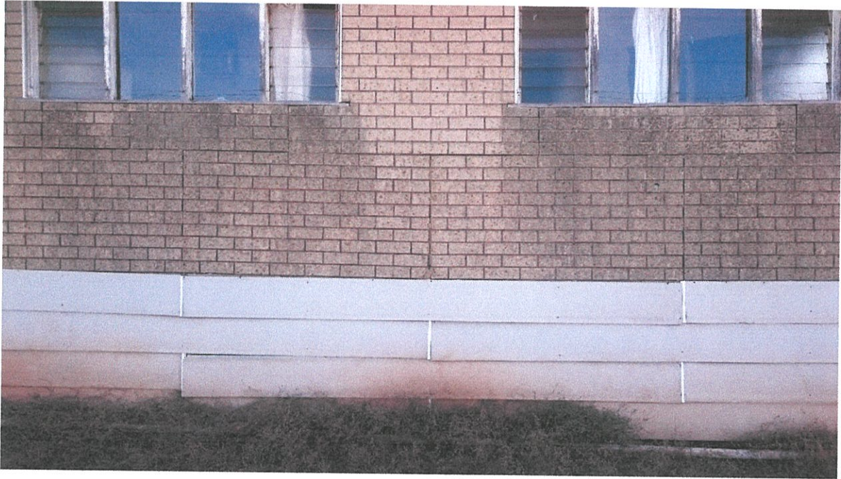
Sagging wall on the Southern side.
