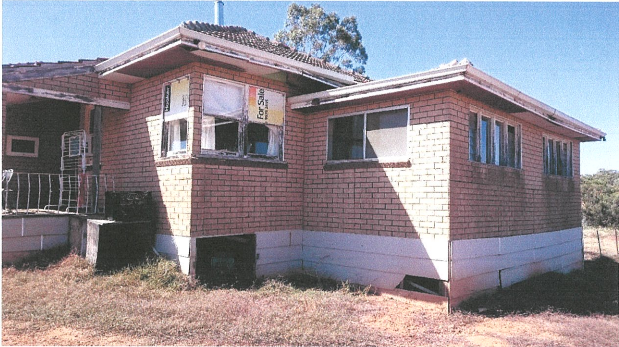
The South Western corner of the house has received the brunt of the weather over the years. Strong winds have blown out windows and eaves. Window frames are nearly rotten.
