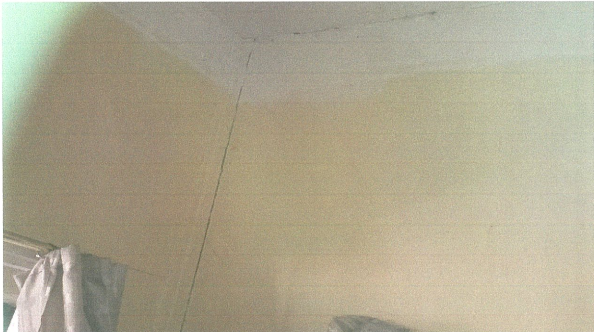
Asbestos sheeting in the laundry cracked at the corner joint.
