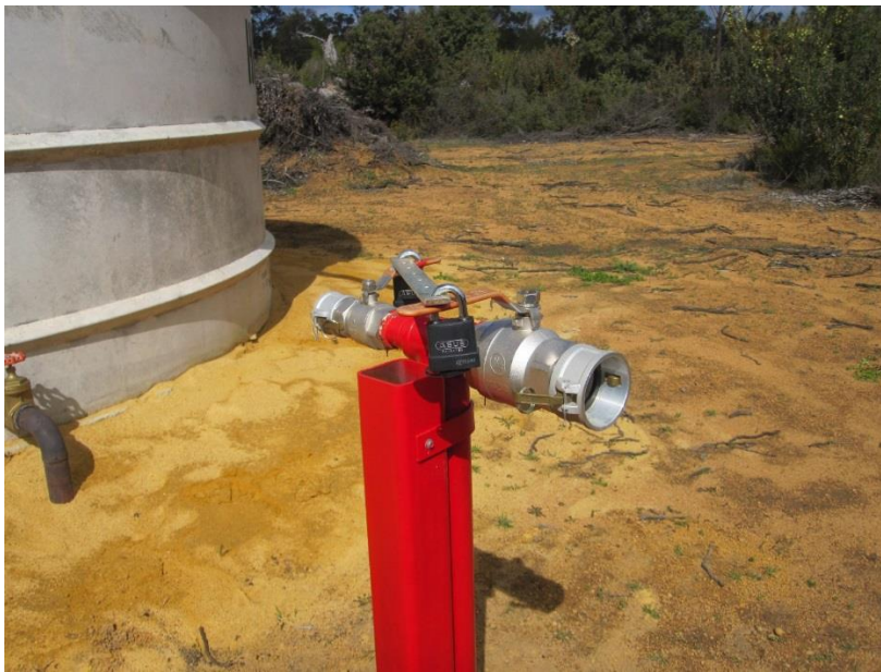
Figure 6. Non-standard fittings installed on Shire water tank in Malkup Brook
