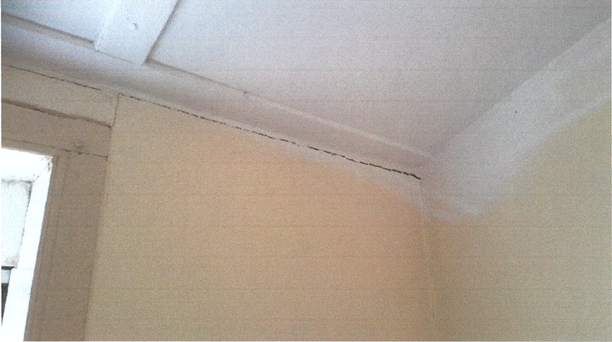
Asbestos cracked in the toilet.
