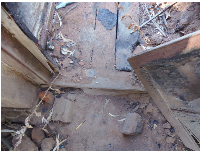
View of remnant material to door threshold.
