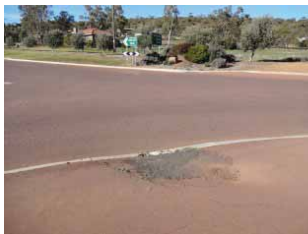
Repairs to paths should be of high quality, providing a smooth surface comparable with the existing path. This path at the corner on Harper Rd needs to be repaired again.
