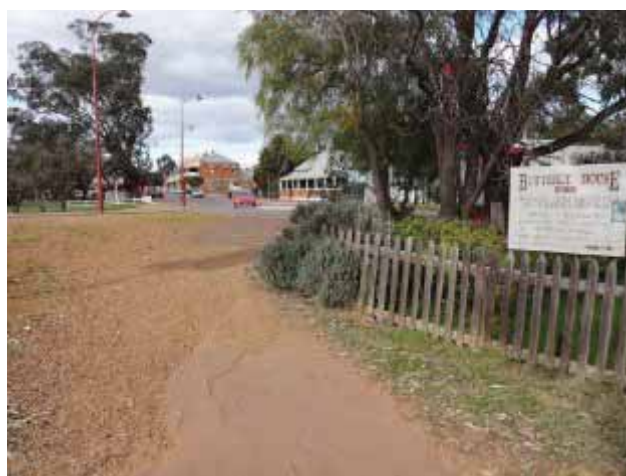
Making repairs to missing pieces of the existing path network will benefit all path users, not just cyclists. This missing section of path is outside Butterfly House on Stirling Terrace.
