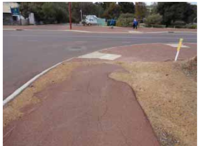
Spot repairs are need to the recently constructed path at the corner of Oddfellow St and Stirling Terrace.
