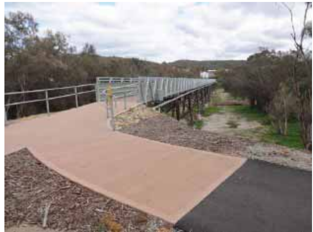
Re-decking the old footbridge over the river and the upgrading of paths either side of the bridge has improved accessibility to the District High School for pedestrians, cyclists and users of other small-wheeled vehicles (such as scooters and skateboards).
