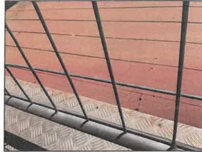
Solid boards already starting to crack
