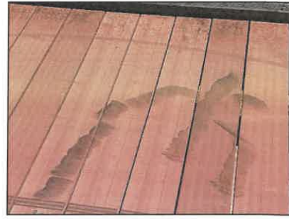
E scooter damage to surface
