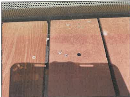
Holes in boards from punched-in screws
