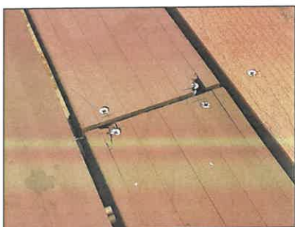
Hollow section construction showing failure
