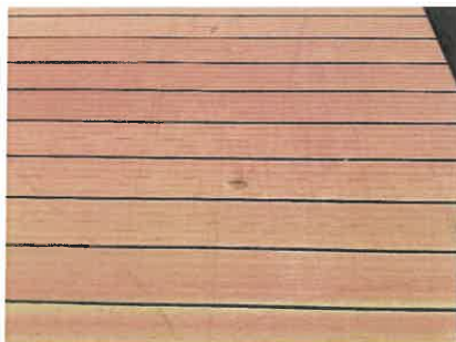
Deep surface damage, including heat damage
