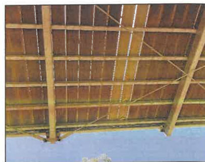
Different board fixings & spacers (coming loose)
