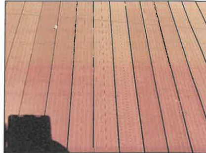
Continuing weathering & board splitting
