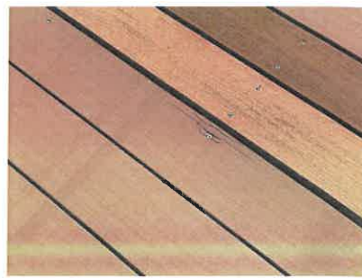
Impact damage on screw line
