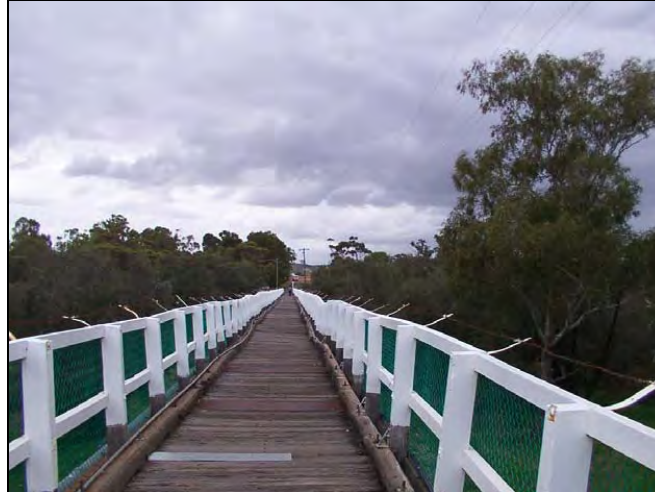
Figure 4 – View of Existing Avon River Footbridge towards Toodyay District High School from Town Centre
