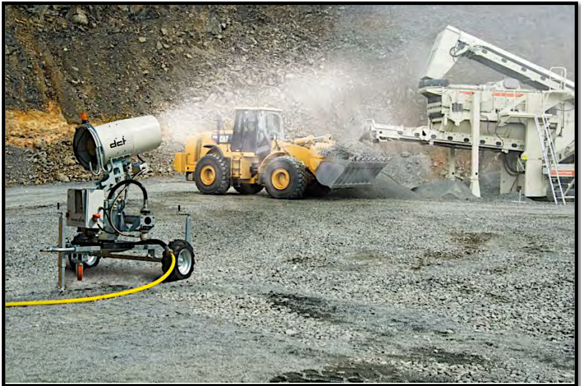
Figure B 3 A large mister that is capturing dust at the drop and loading points of a screen.
