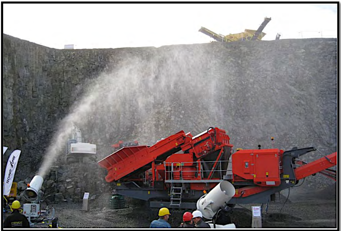
Figure B 2 Misting technology that provides overall dust capture at mobile crushing facilities. The same can be achieved using small misters at drop points combined with wetting down of the hard stand.
