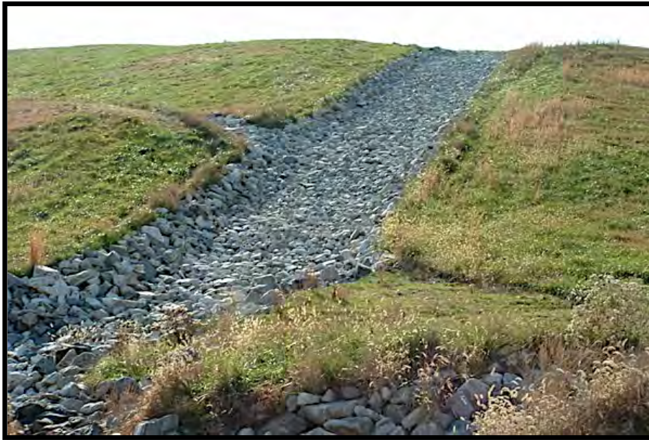
Figure C 7 Examples of rip rap and stone pitching to manage water on slopes, slow the water flows. All detention basins will be provided with rock pitching to protect the outlets
