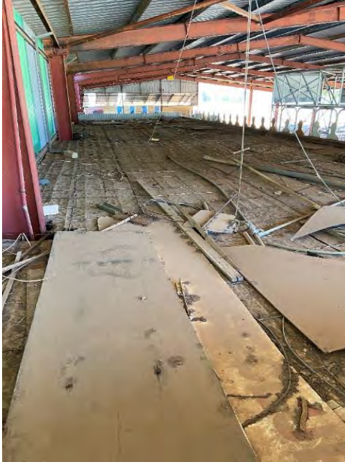
PICTURE 31 – COLLAPSED CEILING
