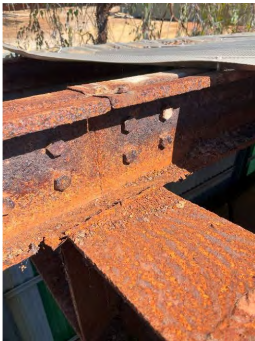
PICTURE 13 – SEVERE CORROSION TO PURLIN
