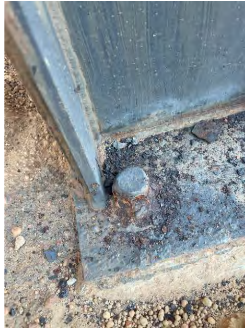
PICTURE 4 – NUT NO LONGER IN PLACE. POSSIBLE SITE WELDING REPAIR HAS BEEN CARRIED OUT
