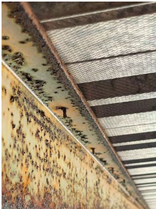
PICTURE 17 - TYPICAL PURLIN CORROSION EXAMPLE
