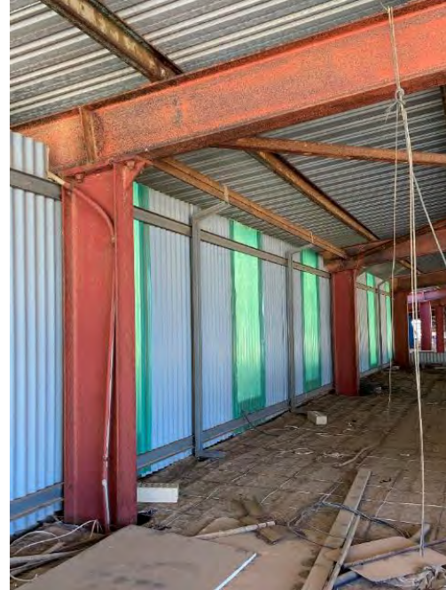
PICTURE 32 – COLLAPSED CEILING
