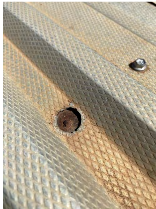
PICTURE 22 – GALVANIC CORROSION AT SCREW LOCATION.
