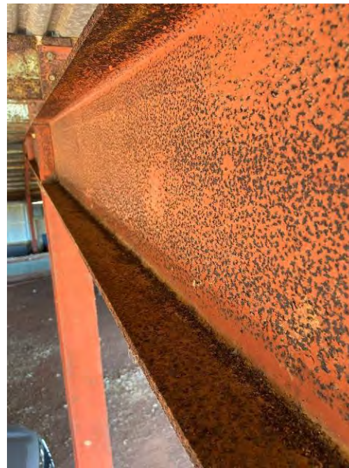
PICTURE 12 - EXAMPLE OF EXTENT OF CORROSION TO STEEL BEAM (TYPICAL)
