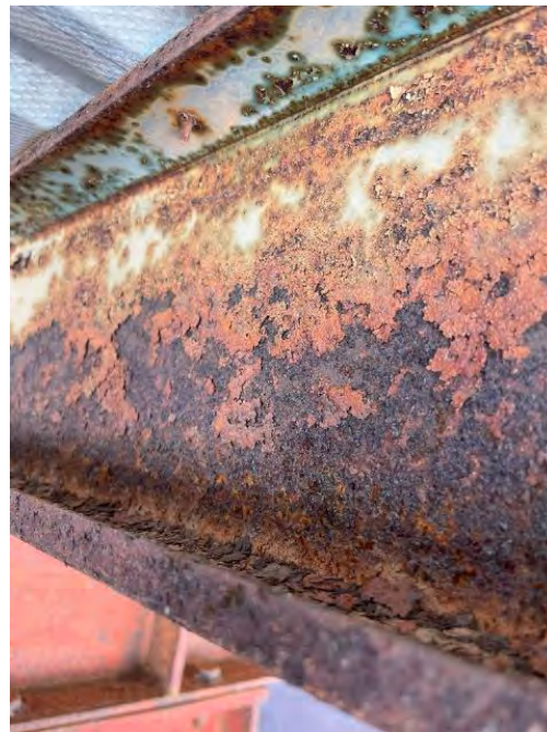
PICTURE 18 - TYPICAL PURLIN CORROSION EXAMPLE
