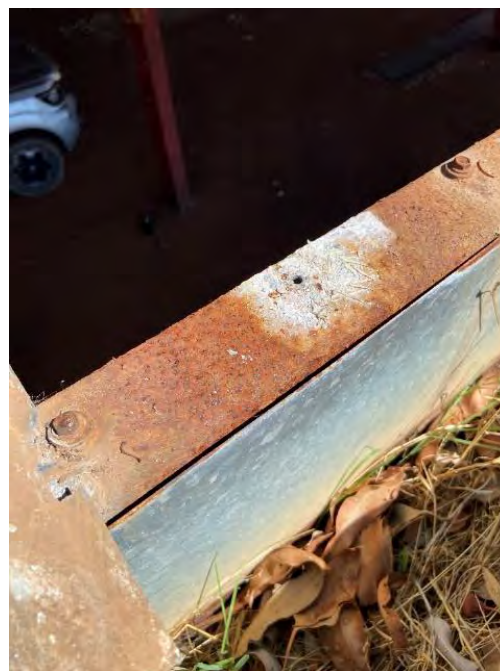
PICTURE 14 – CORROSION TO TOP OF PURLIN (ROOF SHEET MANUALLY REMOVED)
